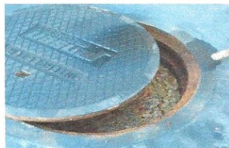
Grease Trap Back-up
